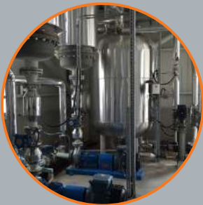
Proses Tank Process Tank
